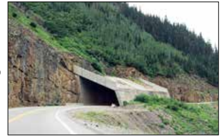
An "overpass" for an active avalanche chute on the Million Dollar Highway, south of Ouray.
